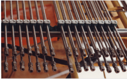
Instrumentation pipework made of stainless steel
